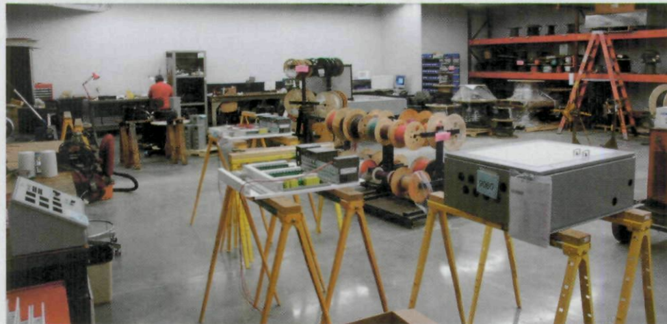
Like adjacent office space, the RC3 plant controls assembly and testing shop has polished concrete floors.
